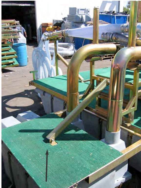
FIG 1N Shown is further detail of foot valve location and brackets.
